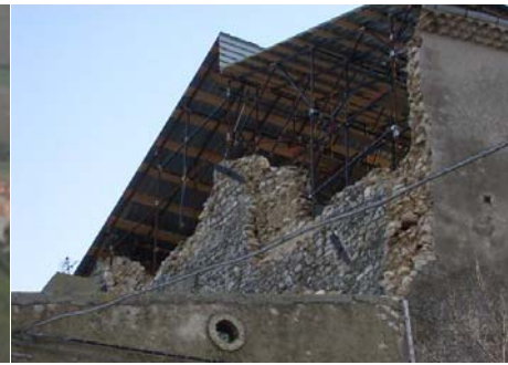
Figure 2. Damage to Marchesale Castle.
